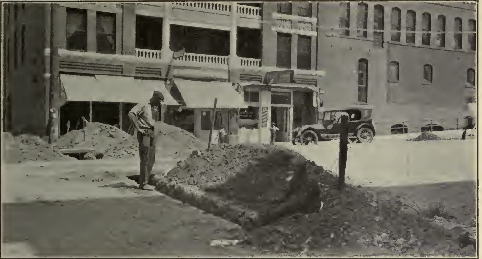
A TYPICAL SCENE IN PRESCOTT WHEN GAS AND WATER MAINS WERE BEING LAID OR RENEWED PRIOR TO PAVING BUSINESS STREETS
